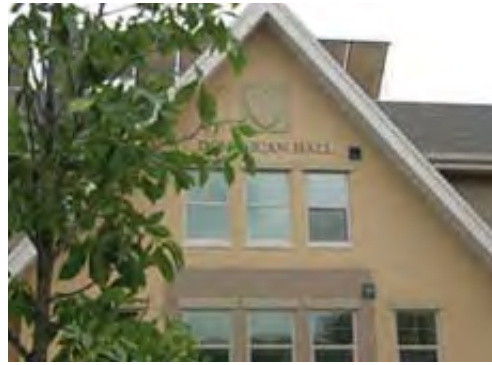
Solar panels on the roof of Dominican Hall reduce energy consumption.
